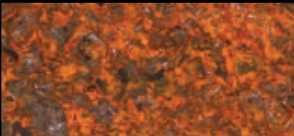
Without corrosion protection treatment
