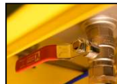
DRAIN VALVE I- CLOSED (HANDLE IN HORIZONTAL POSITION).
