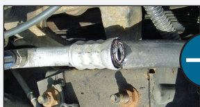
PROBLEM: Damaged A/C hose leaking at connection
