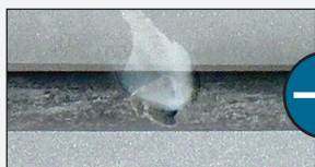
PROBLEM: Damaged A/C aluminum line
